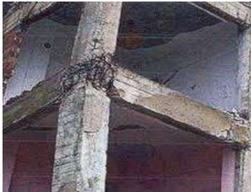
Fig 3: Beam-column joint failure due to different loading condition
